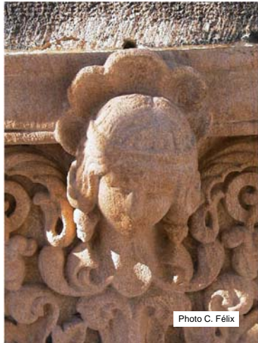
Materials and conservation of built cultural heritage – The weathering of the natural building stones. BR 4/5
