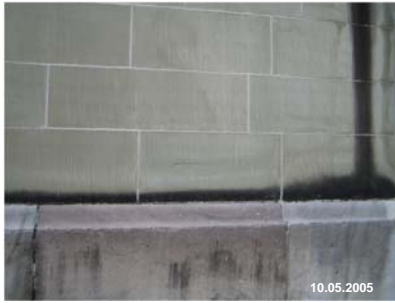
Materials and conservation of built cultural heritage – The weathering of the natural building stones. BR 82
