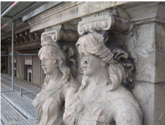
Luzern, former Hotel Bearivage; stone casts dating from ca. 1910
