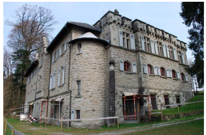
The "economy building" seen from the west with its two largest and most damaged walls in 2009. Lighter stones had their surfaces knocked off mainly in 2005 and 2006.
